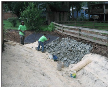
Figure 6.3-21 Rip-Rap Placed by Hand to Reduce Erosion (Source: Anne Arundel County website)
