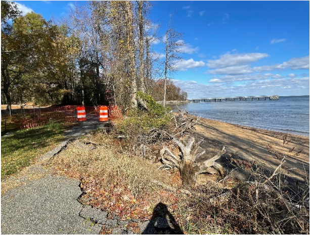
Photo 12 – Path Blown Out behind Narrowest Part of Beach
