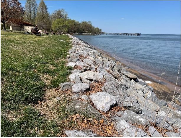
Photo 15 – Stone Slope Protection with Voids
