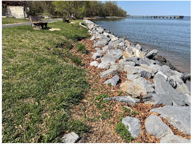
Photo 18 – Multiple Washout Areas behind Structure
