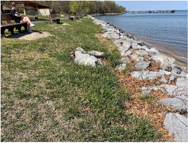
Photo 17 – Stones Pushed back off Structure
