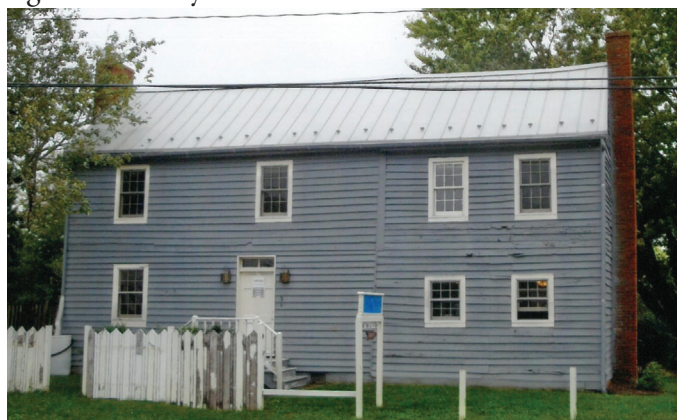
Friendship Parsonage used the County's Historic Preservation Tax Credit to repair siding on the 1825 structure.
