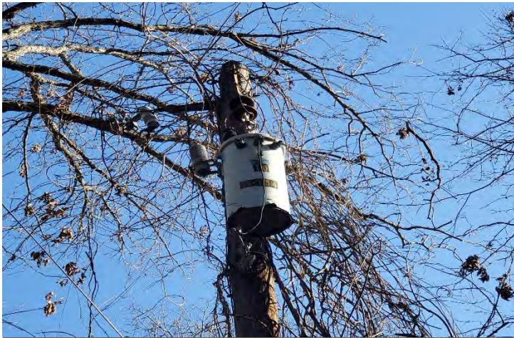
Pole mounted transformer – Southern edge of the Site. Transformer: #85-154 Pole: 24691
