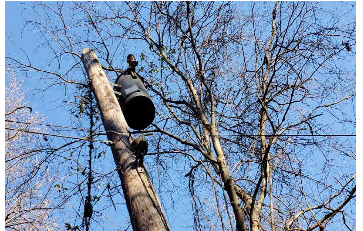
Pole mounted transformer – Southwest portion of the Site
