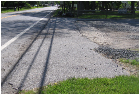
Poorly defined ingress and egress
