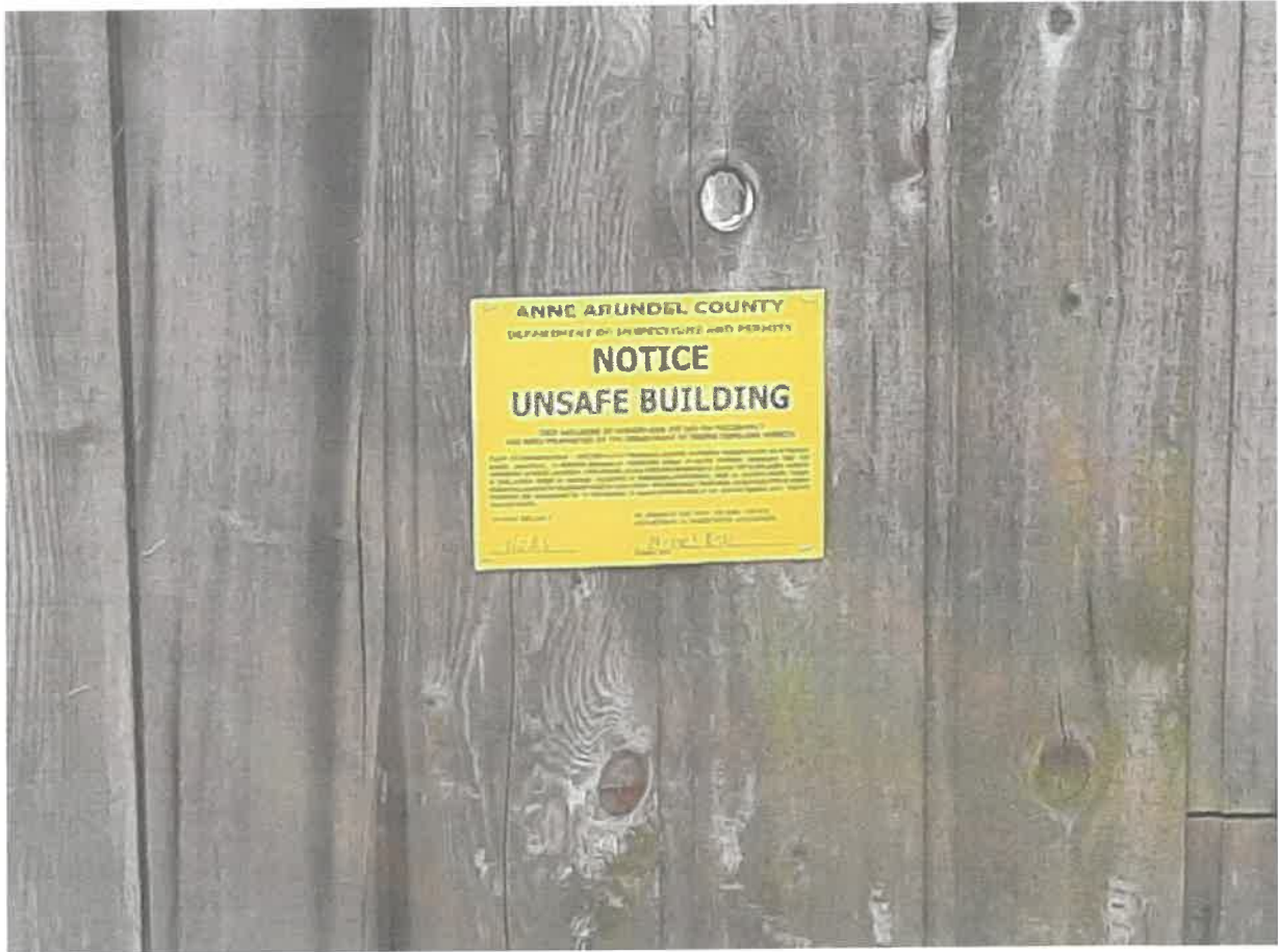
Notice of unsafe building posted at 1702 Vineyard Trail
