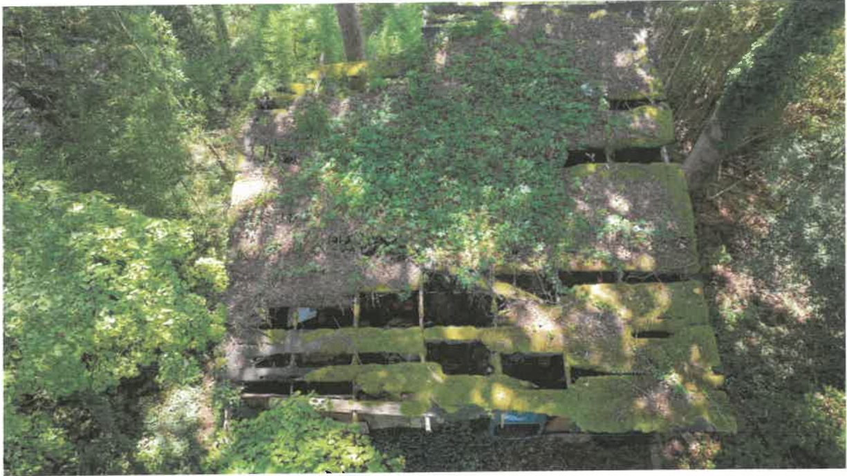
Pictures of dilapidated structure at 1702 Vineyard Trail (aerial and bottom)
