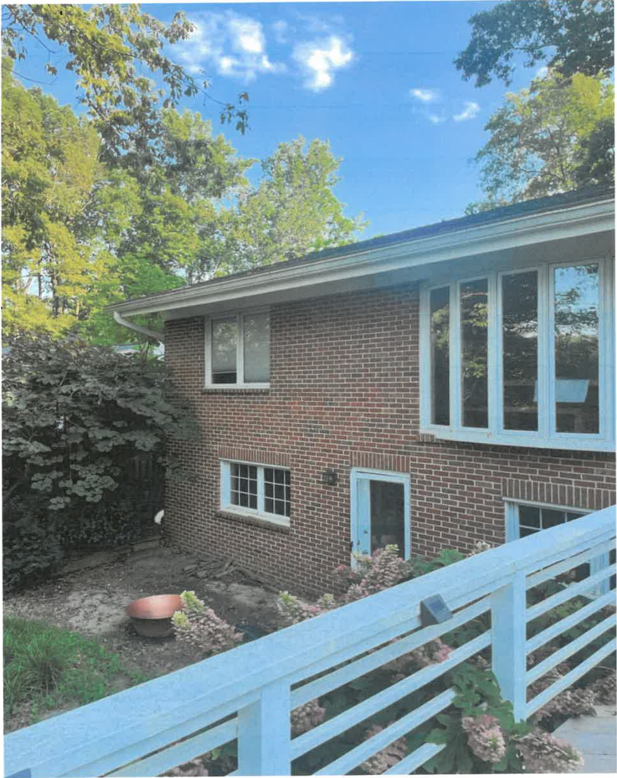
Photo of rear of existing home. Location of proposed 3x8 2 nd floor addition, 4x10 1 st floor deck, and 4x13 2 nd floor deck.
