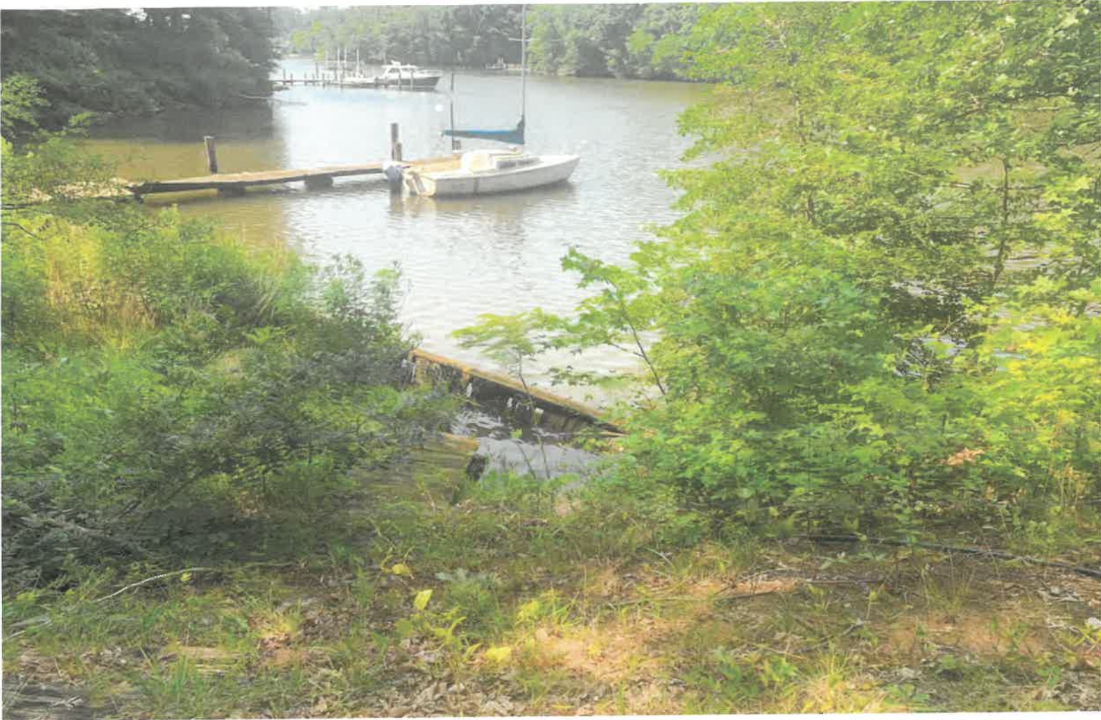
Photo #25 Looking Southwest At Toe Of Slope & Existing Bulkhead, No Erosion Present
