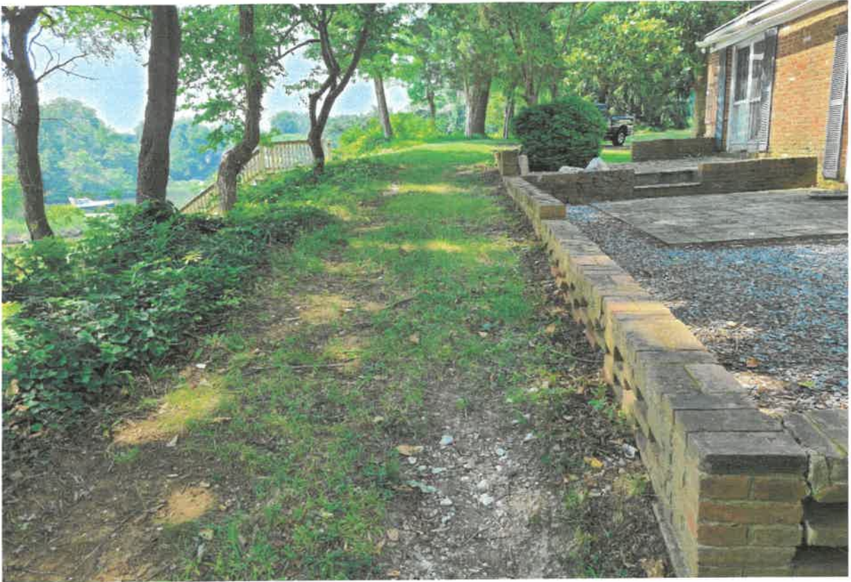
LOOKING SOUTH AT EXISTING EAST SIDE LAWN, BRICK WALL AND GRAVEL SLATE PATIO EAST OF TOP OF SLOPE
