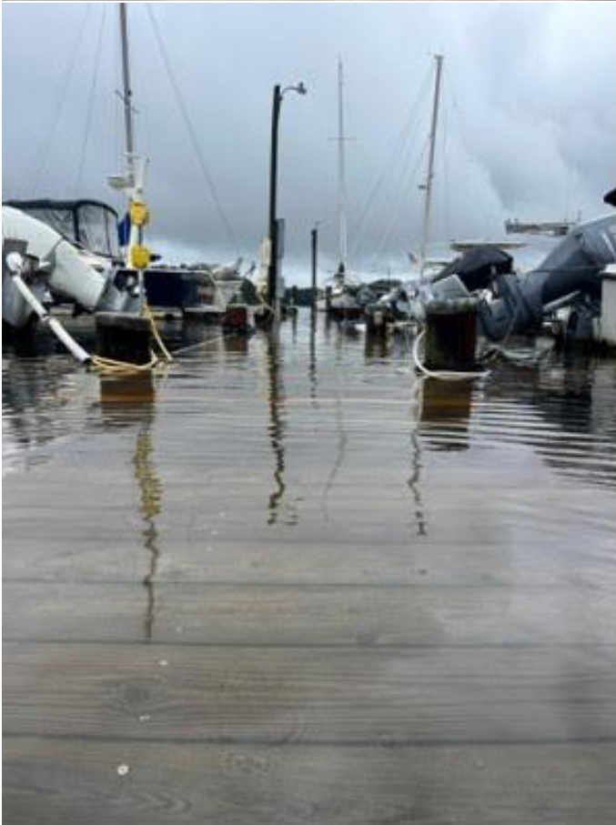
Pier is underwater during storms and surges – occurs 6- 8 times a year and has increased over the years
