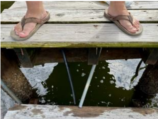
Areas of piers broken off and fallen into water. Hazard tape prohibiting access during repairs. More failing areas each season. The scope of failures are beyond general maintenance such as repairs to singular deck boards or new nails or screws in specific boards.
