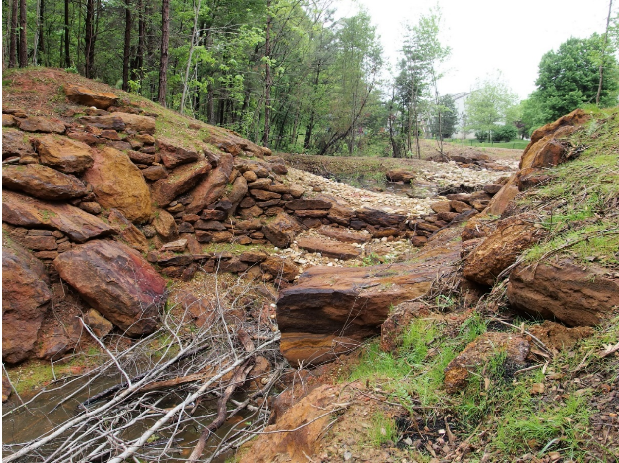
Figure 16: Hospital Drive SPSC, novel cascade weir design to navigate breach in former dam (Anne Arundel County)
