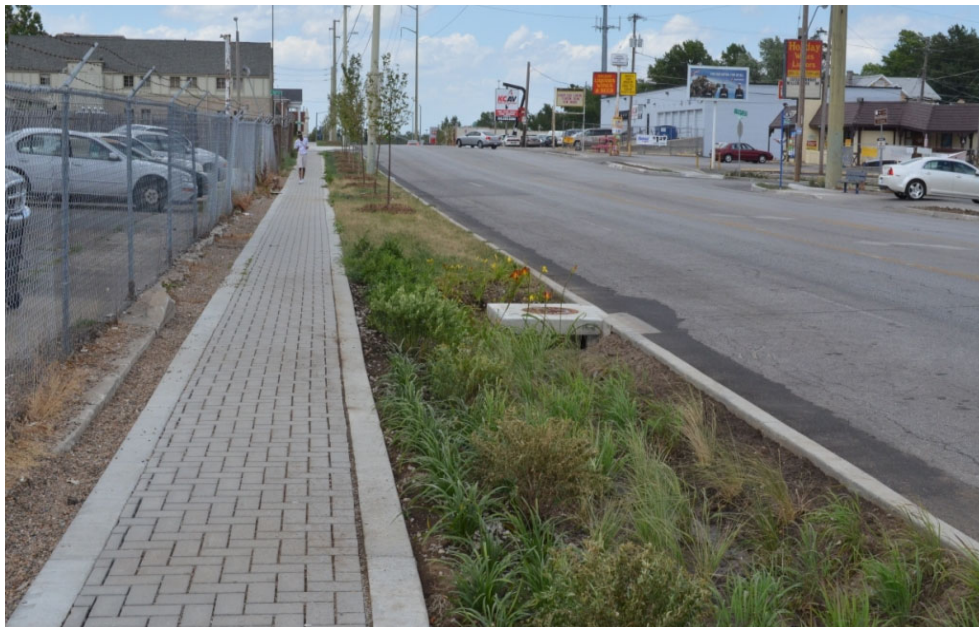
After – Pervious Sidewalks/Improved Vegetation
