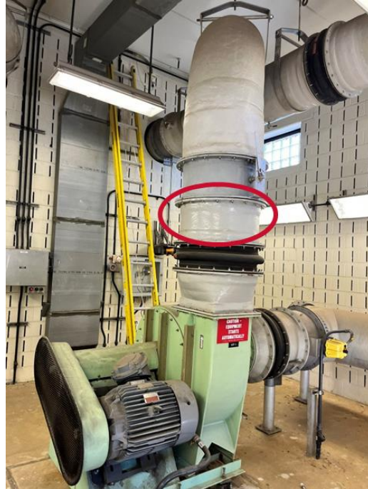
Figure 2-7 Proposed H 2 S monitoring location at the aeration blower facility
