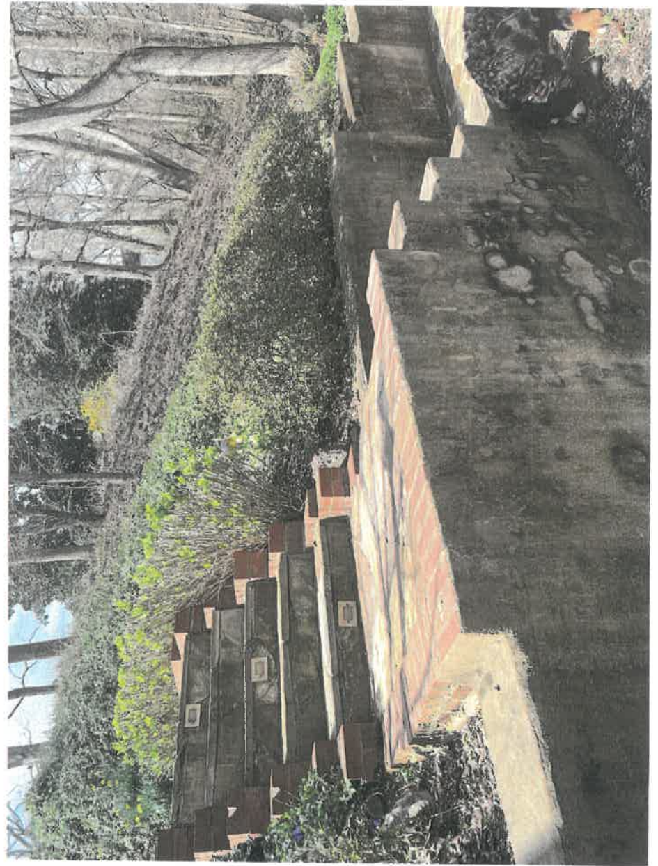
Existing Exterior Staircase - Uneven Riser Heights
