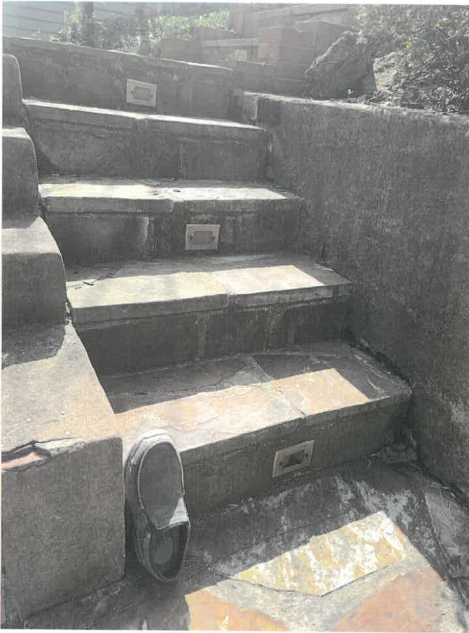
Existing Exterior Staircase - Uneven Riser Heights
