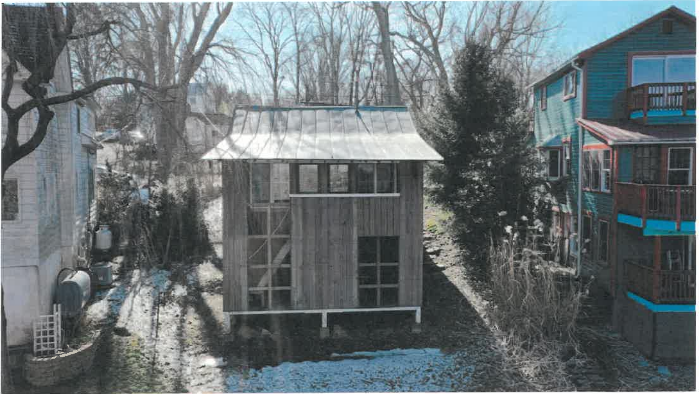
REAR ELEVATION: EXISTING FACADE TO BE DEMOLISHED AND REPLACED WITH NEW FOUNDATION AND LIVING SPACE UNDER EXISTING ROOFLINE.
