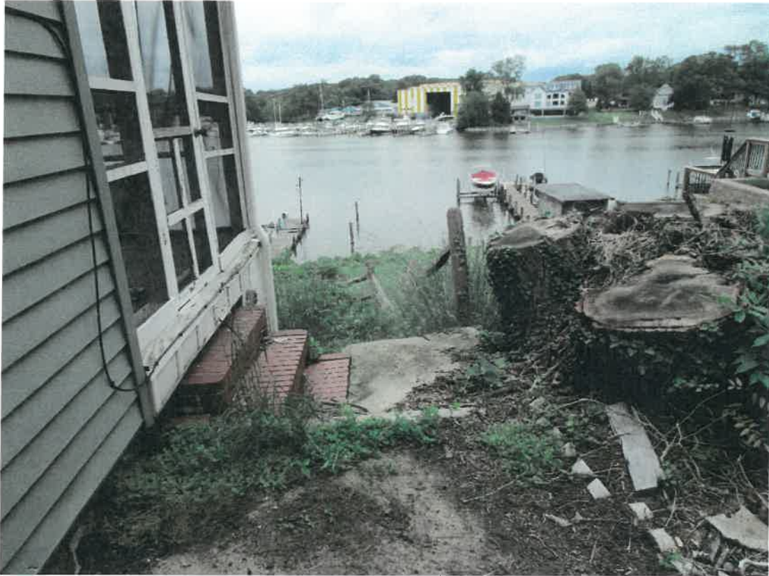
East corner of existing dwelling damaged and remaining hardwood tree cluster stumps.
