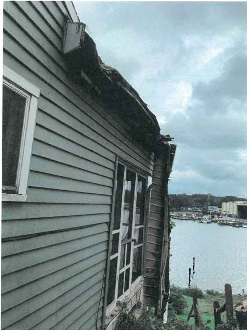
East corner of existing dwelling damaged roof.
