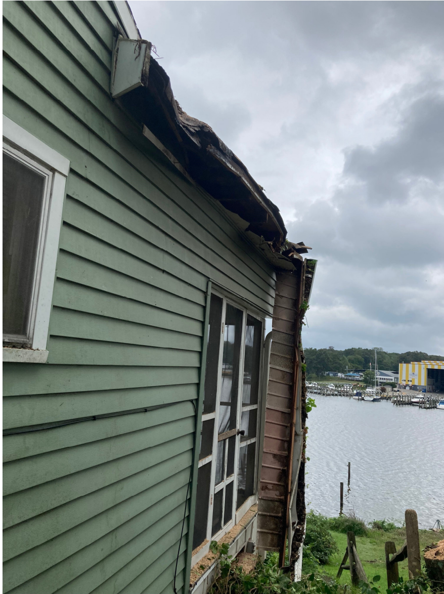
East corner of existing dwelling damaged roof.
