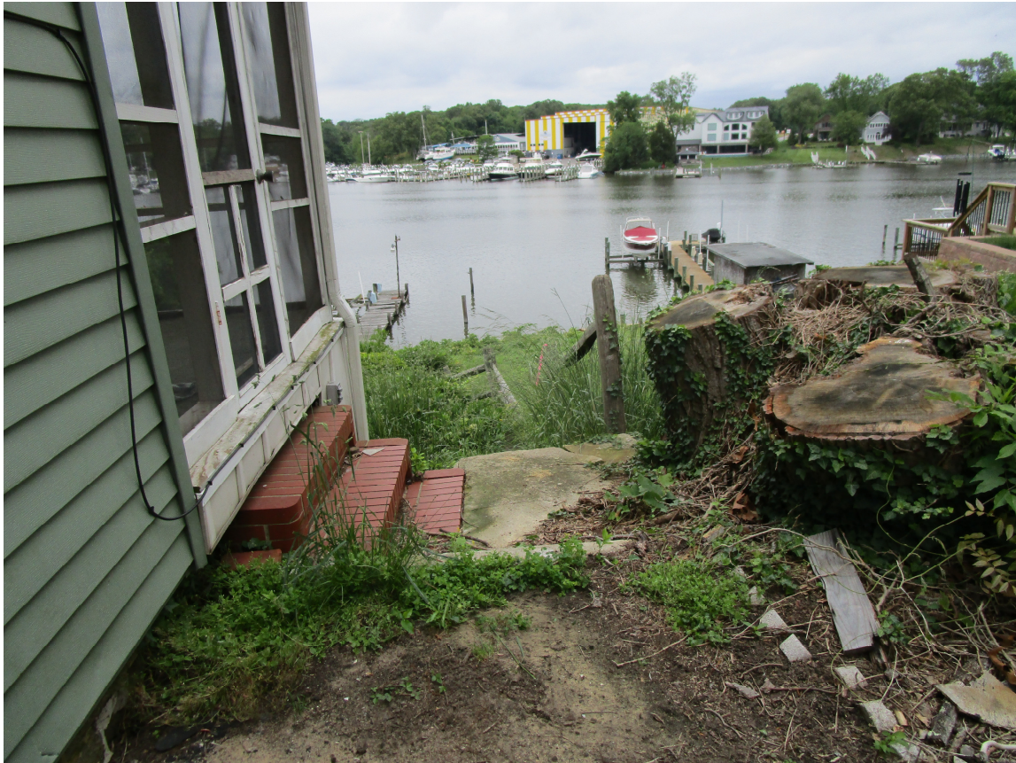
East corner of existing dwelling damaged and remaining hardwood tree cluster stumps.
