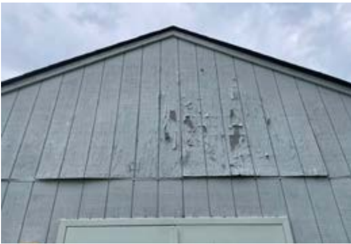
Figure 24. Chipping paint on front of greenhouse
