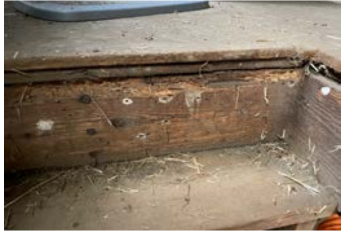
Figure 20. Second floor landing has visible damage Source: AECOM
