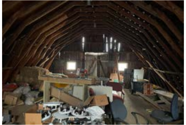
Figure 17. Second floor of barn is used for storage and has visible exposure to the outside
