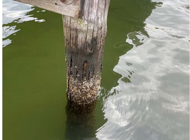
Photo 6 – Piling necking at the waterline
