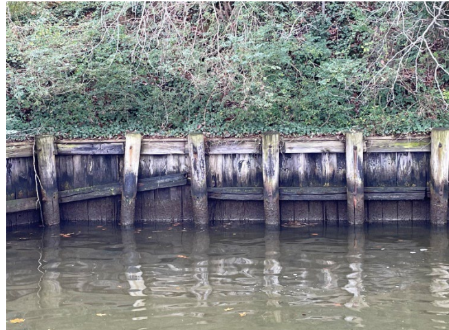
Photo 2 – Deteriorating bulkhead members
