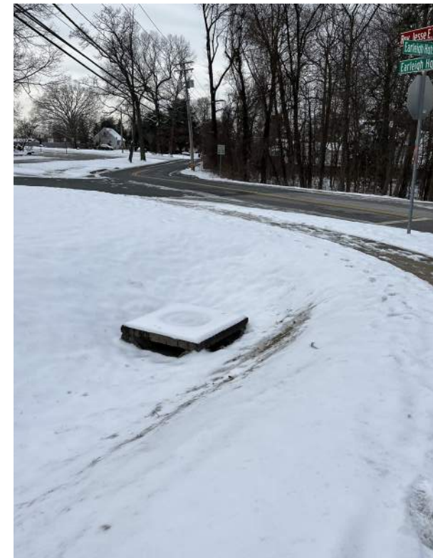
Figure 23. Existing drainage structure on Earleigh Heights Road
