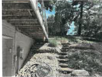
6. Boulder Stairs to Cantilevered Entrance Deck Adjacent to Garage Doors - Looking South
