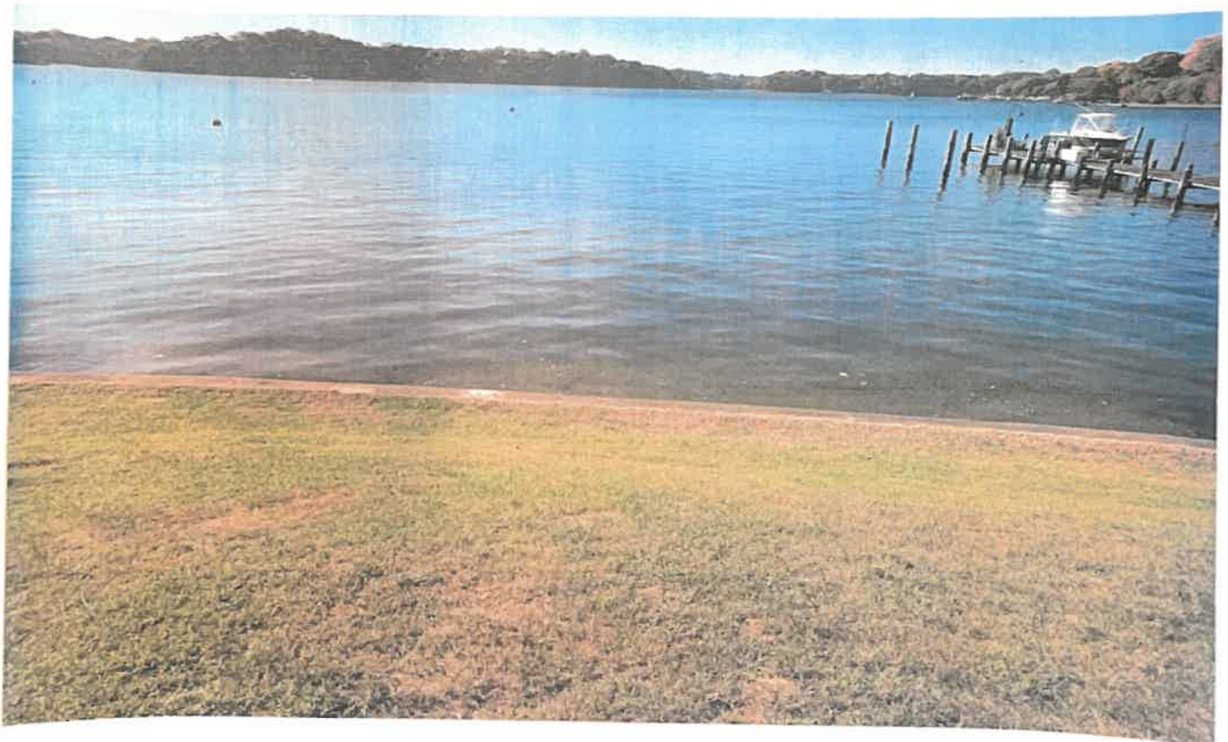
Photo Location #9 Looking West Towards Toe Of Slope, No Erosion Or Channelization Present
