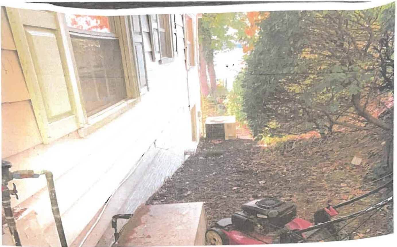
Photo Location #16 Looking West Down Slope, Area In Good Condition With No Erosion Present
