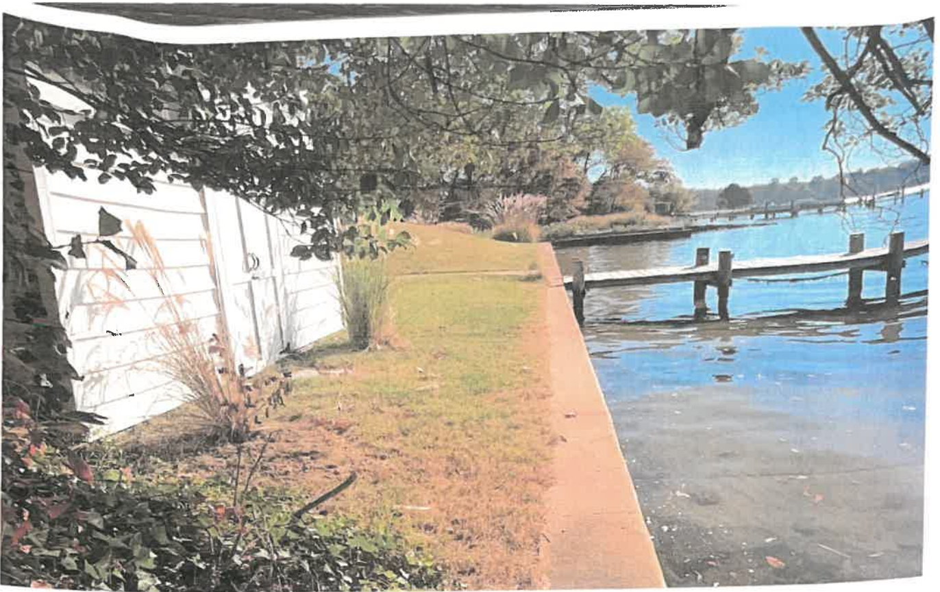
Photo Location #10 Looking Across Bulkhead Towards Toe Of Slope, Area Stable With No Erosion Or Sediment Present
