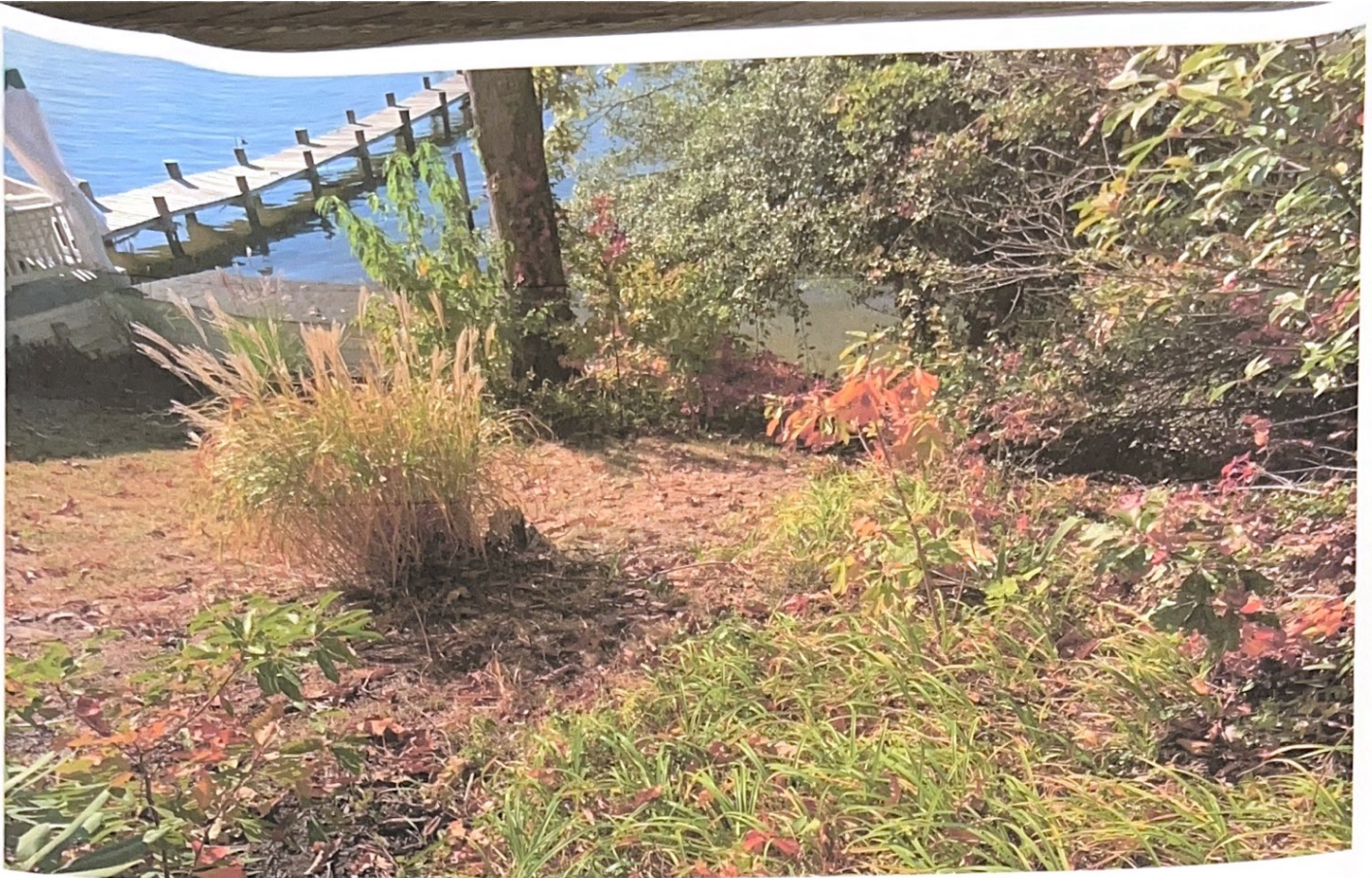
Photo Location #13 Looking West Down Slope, Area In Good Condition With No Erosion Present
