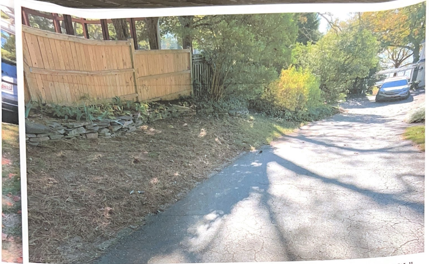
Photo Location #2 Looking Southwest Towards Existing Steep Slopes, Stable With Vegetation & Existing Flagstone Wall
