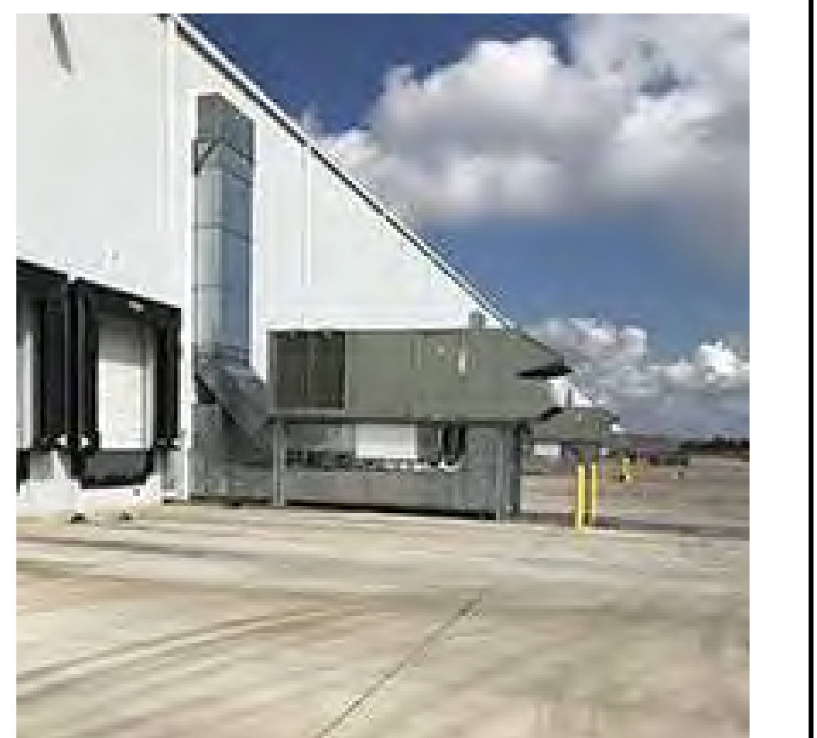
PHOTO OF EXAMPLE GRADE-MOUNTED ROOFTOP UNITS (RTU)
